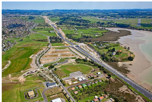
Figure 7 – SH18 Hobsonville Deviation under construction passing through Auckland's Northern Strategic Growth Area
