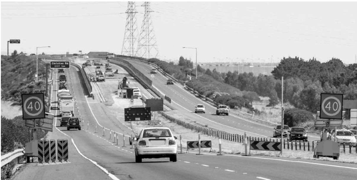
Photos 1 & 2: Trailer Mounted EVSLS's on site
