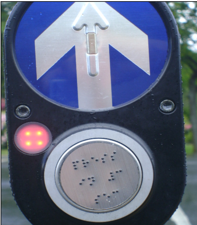
Figure 4 -Red LED indicating longer crossing time chosen and braille label advising 'Hold for 3 sec'
