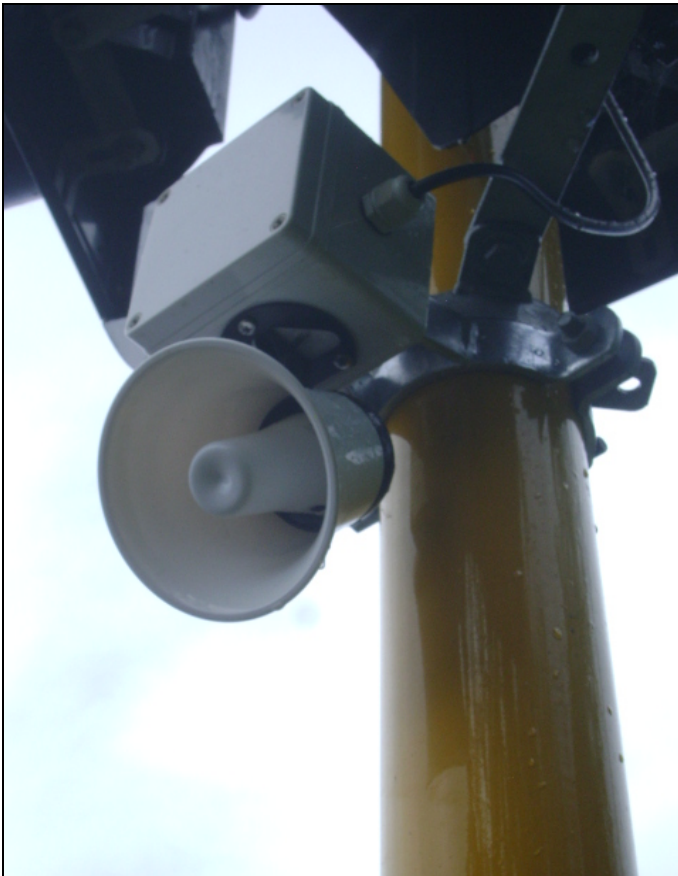
Figure 2 - DPCS Audible Voice Message Unit which announces to pedestrians that a longer crossing time can be chosen, if they need it, by holding the button in until it beeps and red LED activates
