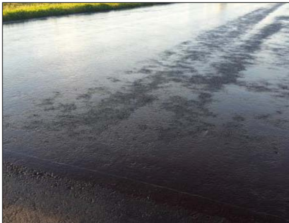
Figure 6: GSB-88 Percolating Into Voids
