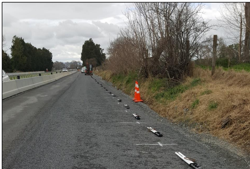
Figure 8 Temporary steel barriers used to increase productivity and create a safer workspace
